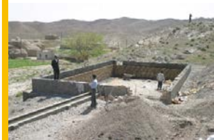
The restoration of a Qanat and its open storage tank (a "Drops for Life" Project)
